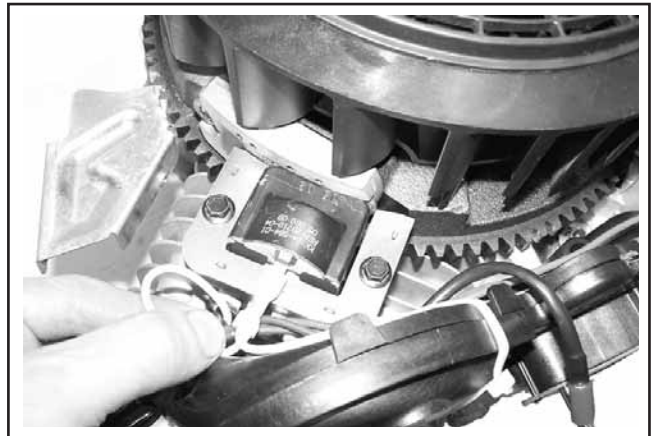
Figure 10-59. Connecting Kill Leads on Fixed Ignition Modules.
